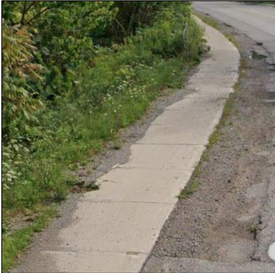
Figure 4c - Sediment Deposits on Sidewalk (south portion, east side looking south)
